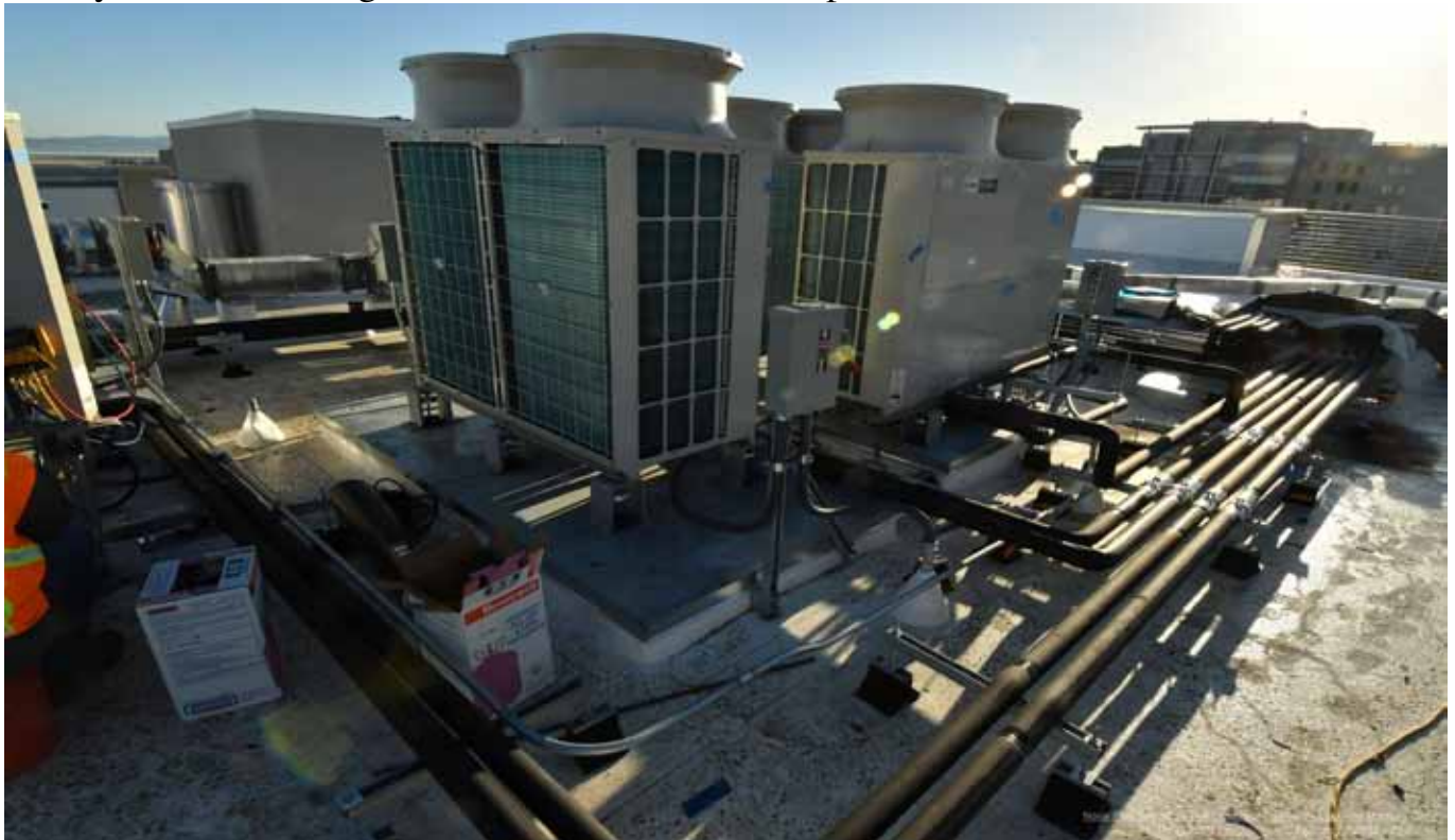
Roof top HVAC unit start up underway
