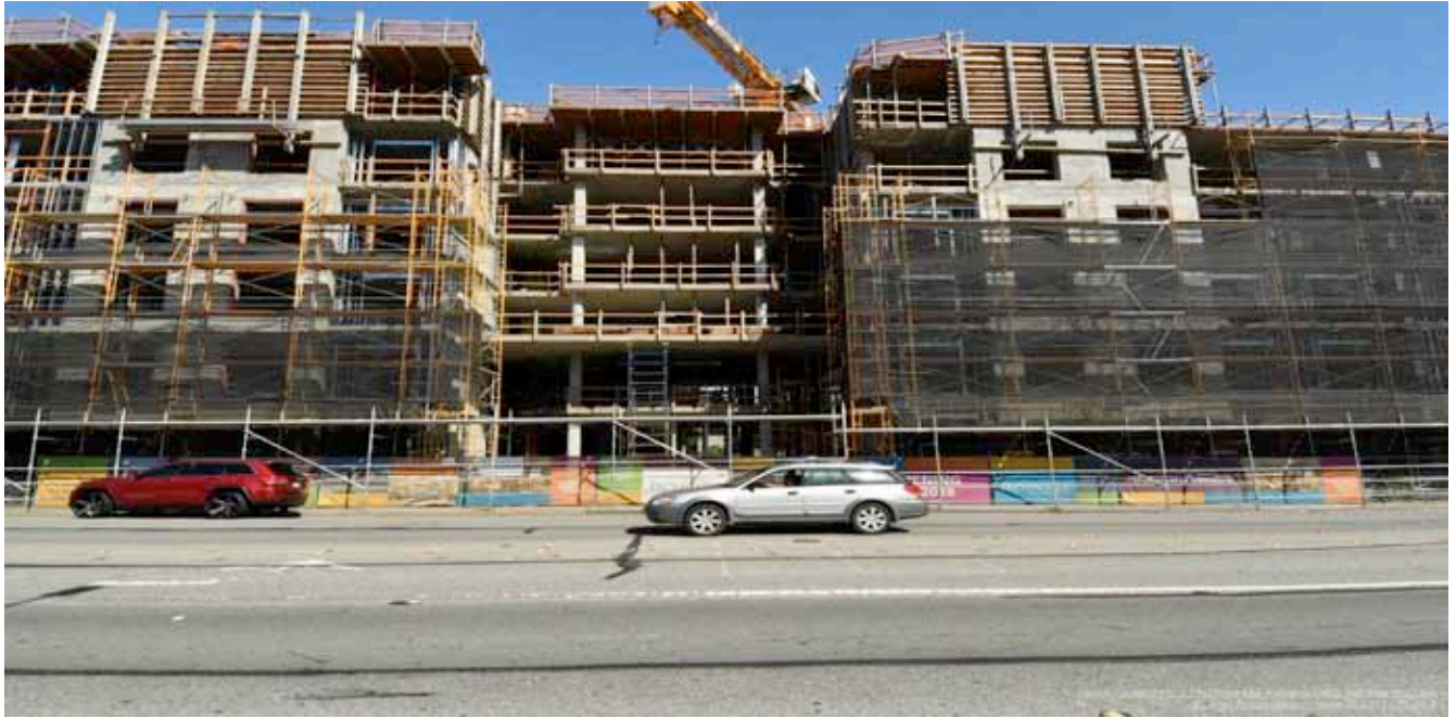
South Elevation of building. Exterior Framing 95% complete and scaffolding being installed to floor 6.
