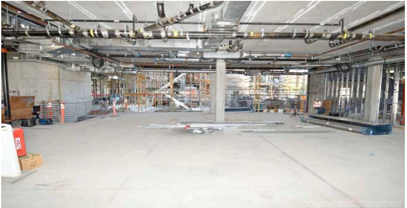
Floor 1 Kitchen/Dinning room looking to the north. All overhead M/E/P systems are now complete.
