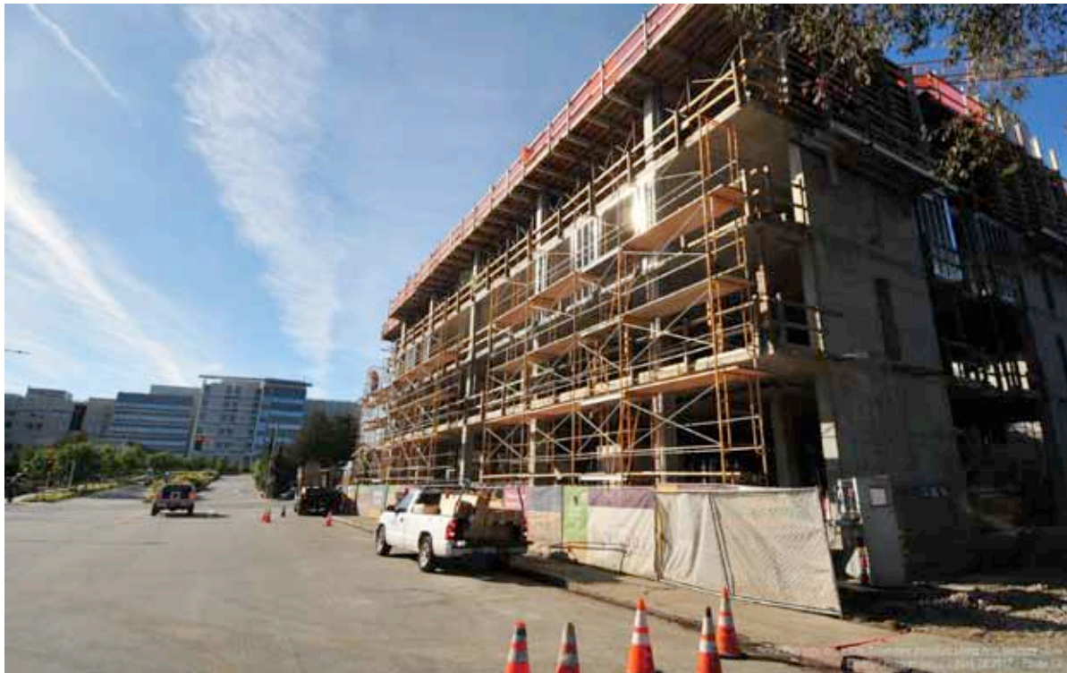
Looking to the North down Magnolia. Scaffold installed on east elevation with floor 3 framing underway.
