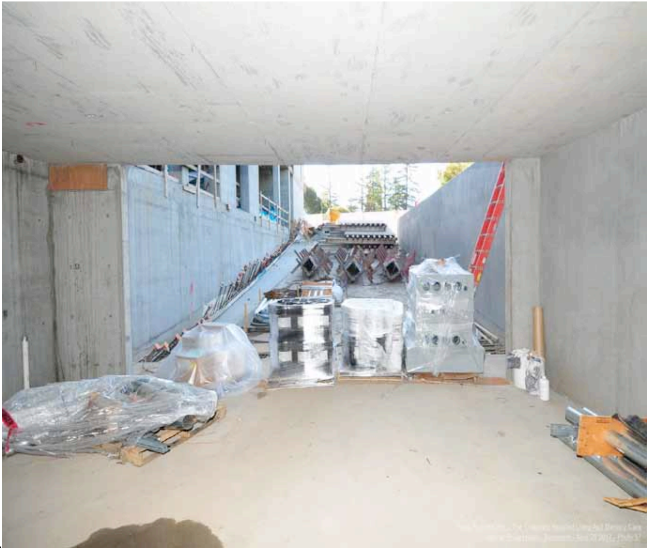
Basement ramp walls complete. Patio slab above complete waiting to pour ramp concrete.
