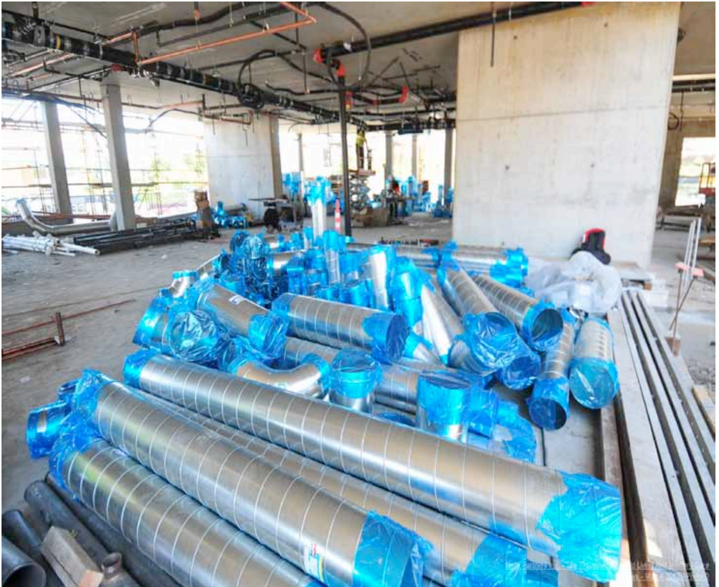
Floor 2 interior overhead Mechanical Ductwork getting ready for installation. Overhead electrical and plumbing systems being installed.
