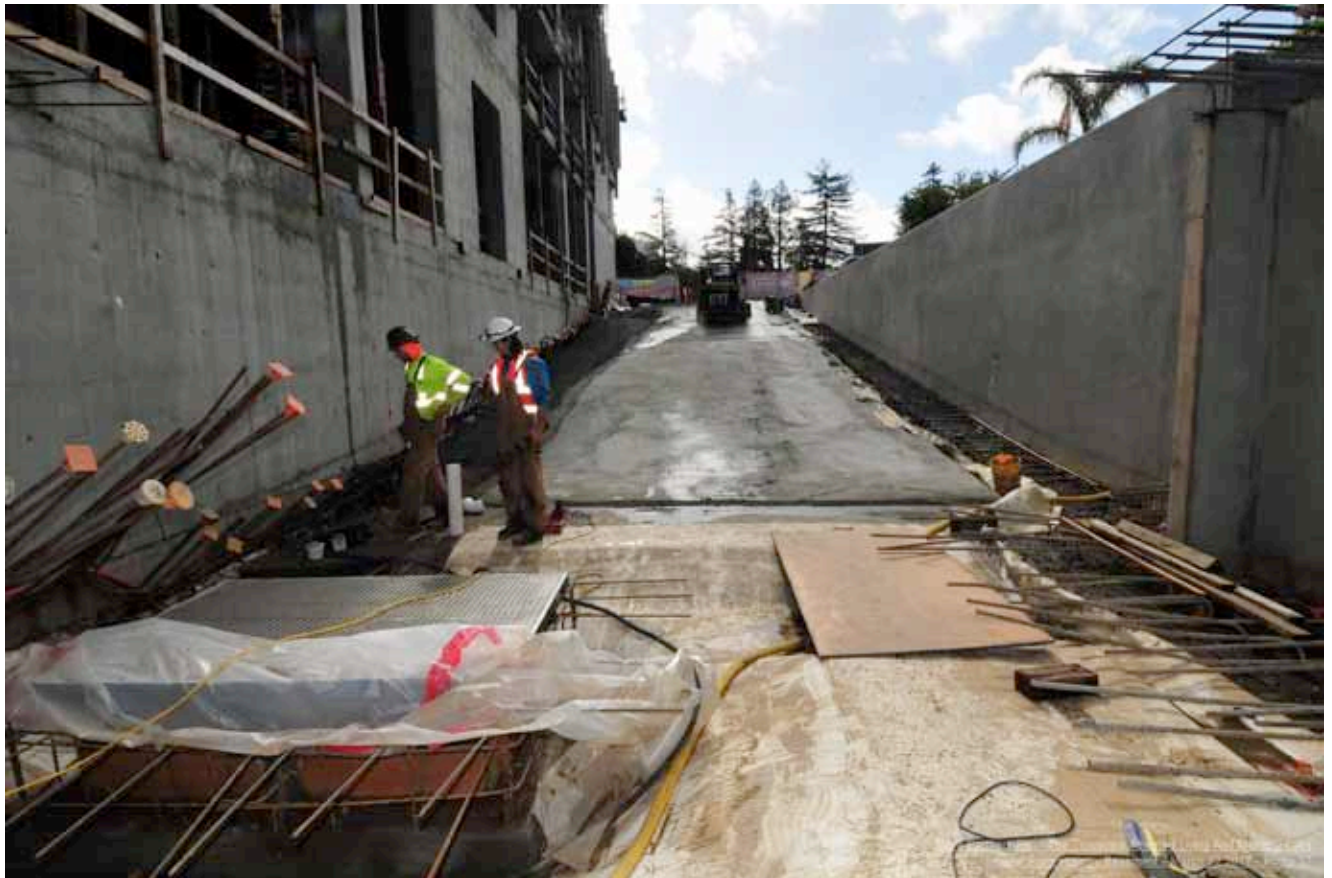
3/31/17 – Basement mud slab poured/ramps complete getting ready to form ramp slab in May
