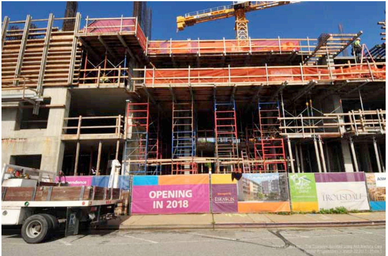
3/31/17 – Looking north into the entry lobby – Scaffold going up ready to pour fourth floor east
