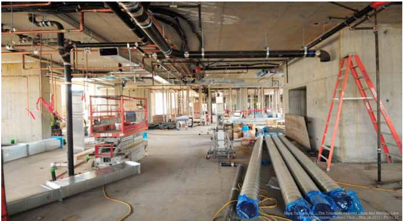
Floor 1 interior Mechanical/Plumbing and Electrical overhead systems being installed and approximately 50% complete.
