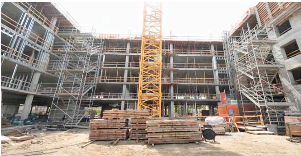
Interior courtyard scaffolding currently being installed. Exterior building framing has begun at all levels.
