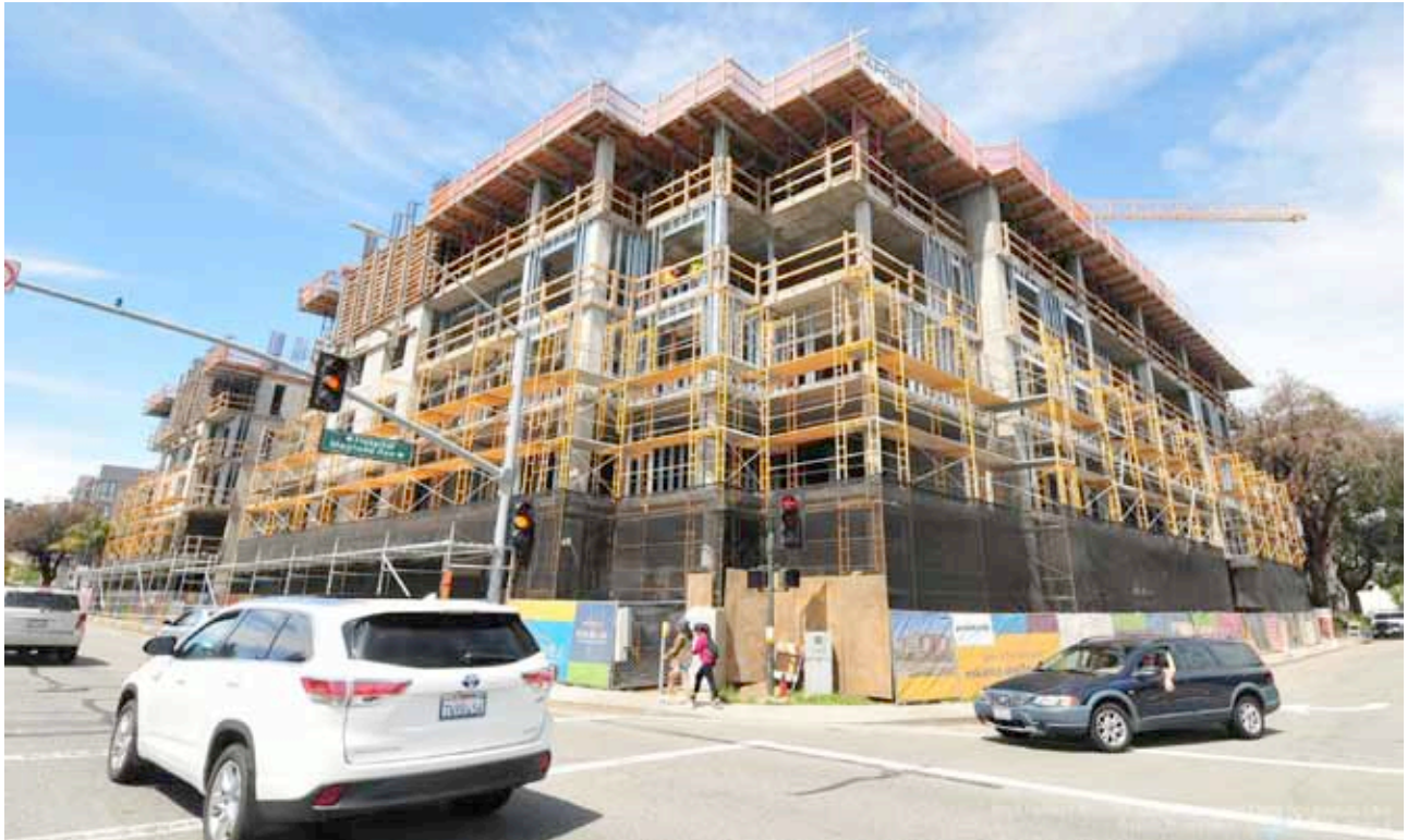
Corner of Trousdale and Magnolia looking to the North West. Scaffolding going up and exterior framing on going.
