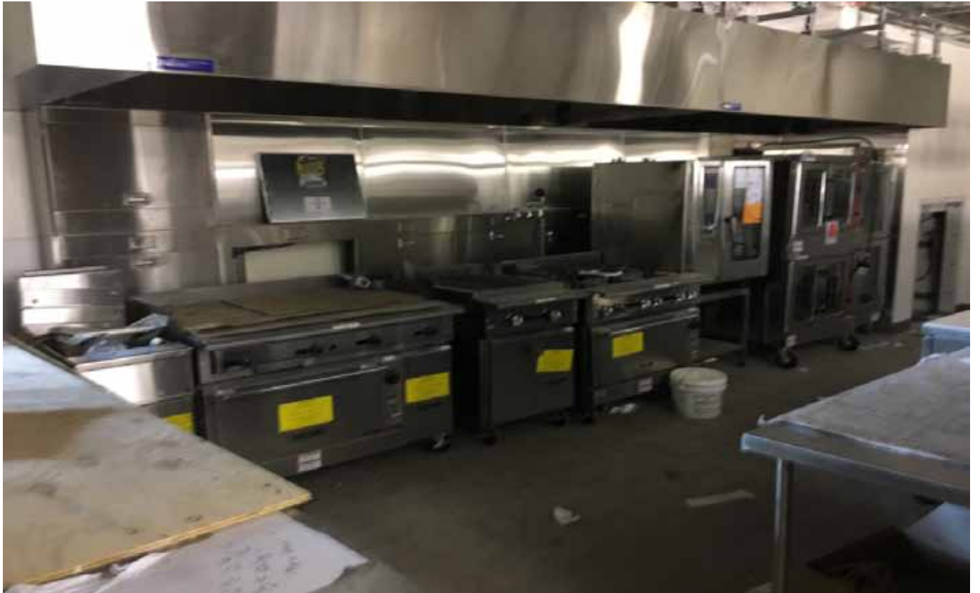
Floor 1 Kitchen Equipment installed
